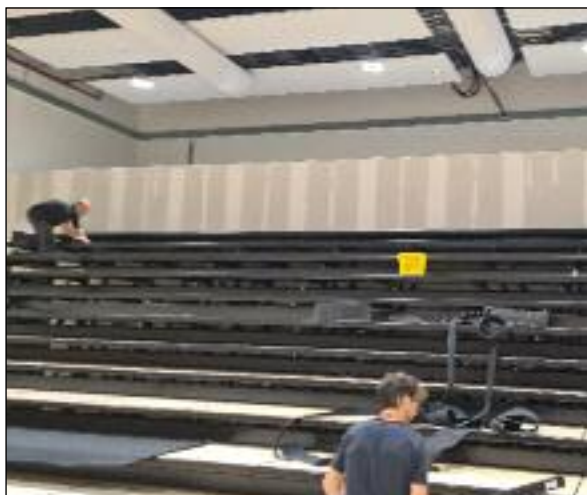
GETTING THERE: The installation of the tiered seating and associated structure has not been straightforward.
