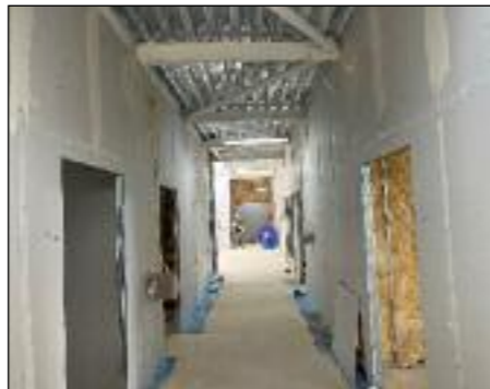
TAKING SHAPE: Block One of Cambourne's extensive construction project is set to be ready for September.
